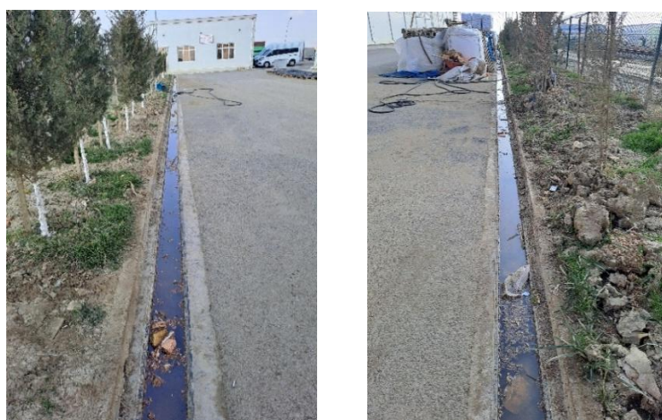
Figure 4 Localized water ponding
